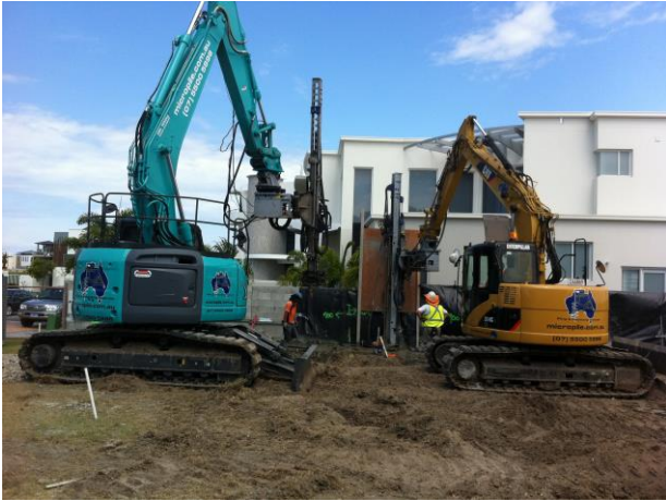
Two drill rigs were used. One was used to install the grout columns while the other installed the 6m long universal beams
