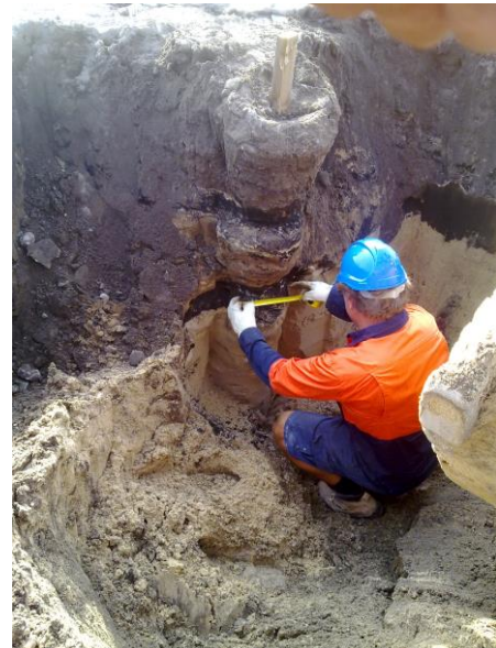
Exhumed test pile where pressure and flow rates were adjusted to determine the change in pile diameter
