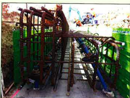
A-frame micropile structure under construction, showing the tops of the rows of vertical and raked micropiles and the reinforcing cage for the concrete capping beam
